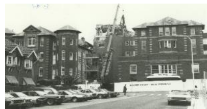
Earthquake damage to the North and York wings of the old Royal Newcastle Hospital, Australia – c.1990
